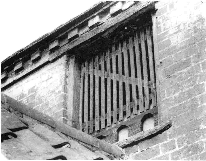
FIG. 130 – At Little Bealings this inserted aperture dates only from the introduction of the small-scale keeping of ornamental pigeons in the late 19th or early 20th century. Earlier the pigeons would have entered at a louver on the apex of the roof.
