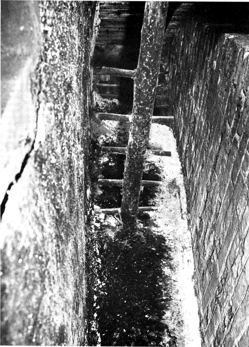
Looking steeply upwards into the front of the chamber, showing a rack made from a round pole (with one peg broken) supported in the wall of the chamber. The outer surface of the brick chimney is unsooted because a layer of daub has been removed during re-pointing, leaving the walls of the chamber undisturbed.
