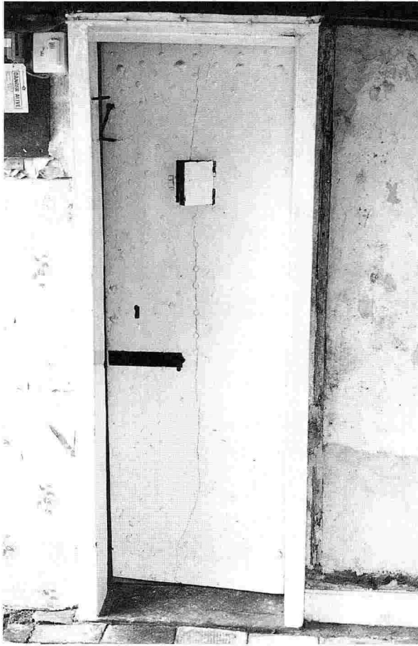
FIG. 146 – The original studded cell door with its inspection window, locks and bolt. The front is made from a single plank on oak 25 inches wide ( photo: author ).
