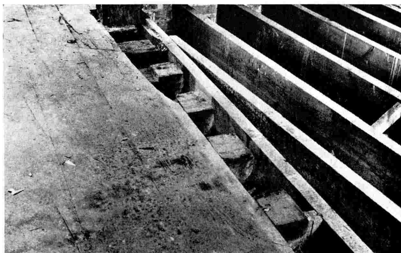
b. The ends of joists, at the northern end of the east range, indicating a first floor overhang. These joists were made visible during the repairs of 1934-5 when this photograph was taken, before being again covered over.
