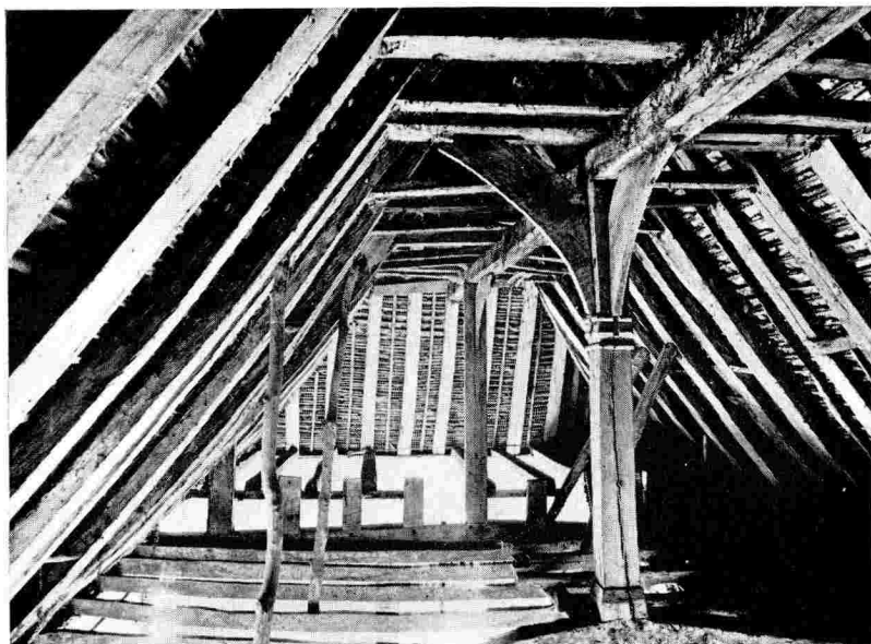
a. The roof-structure over the east range looking south, showing the open truss No. 7 and, beyond, the closed truss No. 8.
