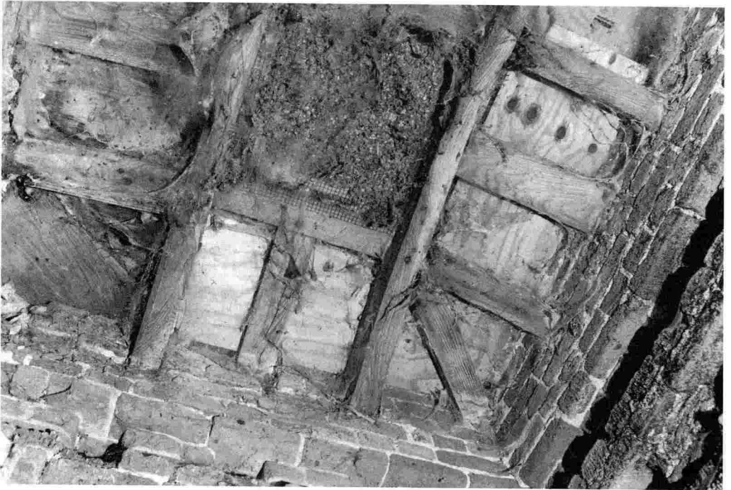
Fig. 5 – The roof structure from below, showing the rectangular aperture through which the pigeons formerly entered ( photo: author ).
